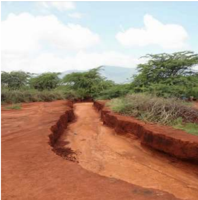
Plate 2. Severe gulley erosion at Mkwajuni village, Lake Jipe leading to severe sedimentation in the lake.
